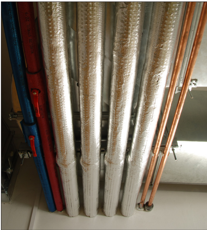
Figure 2. The self-drying insulation in the HVAC laboratory in Brno
