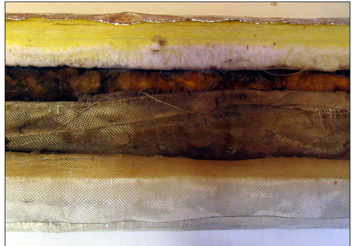
Figure 8. Frost deposit in the insulation when freezing temperatures occur; in this case, the piping was below zero
