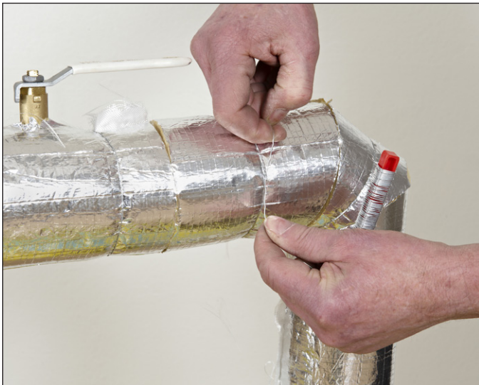
Figure 6. The pipe section with the manufacturing-applied fabric wick can be then placed into its position
