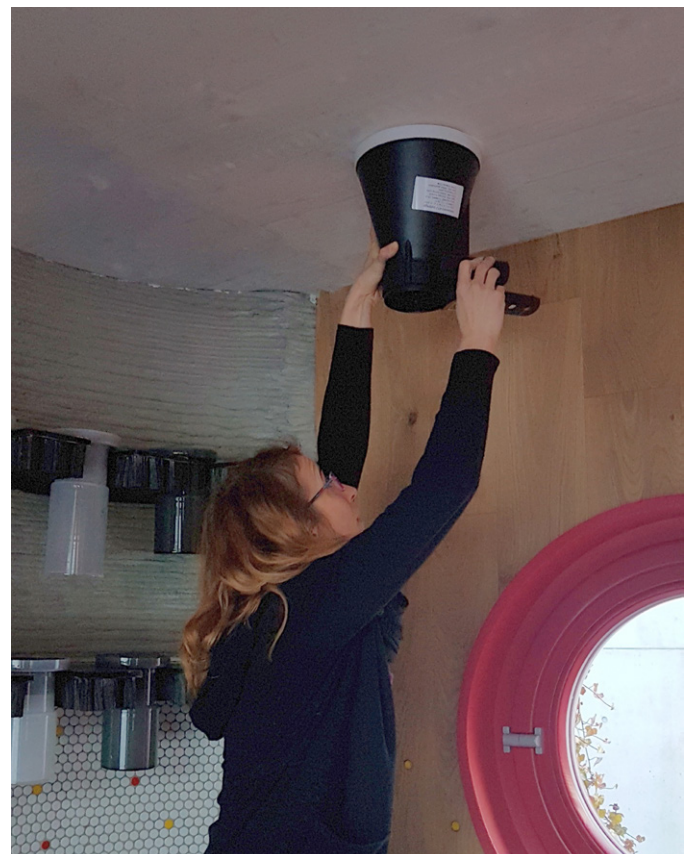
Figure 4. Verification of the air flow at the exhaust of the ventilation system [photo authors]
